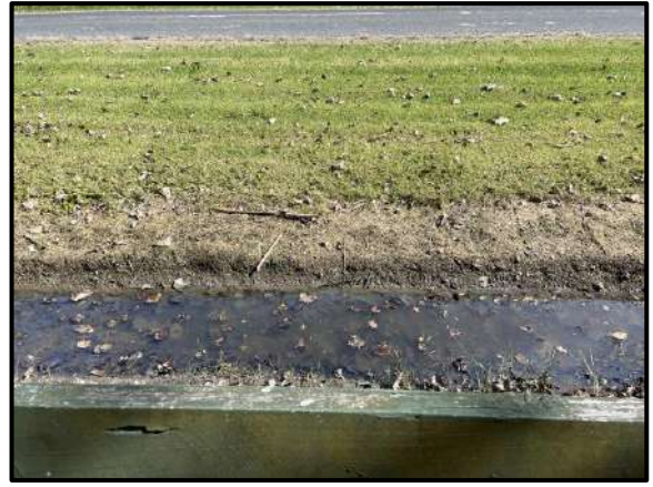
Photo 4: Standing water in drainage channel.
