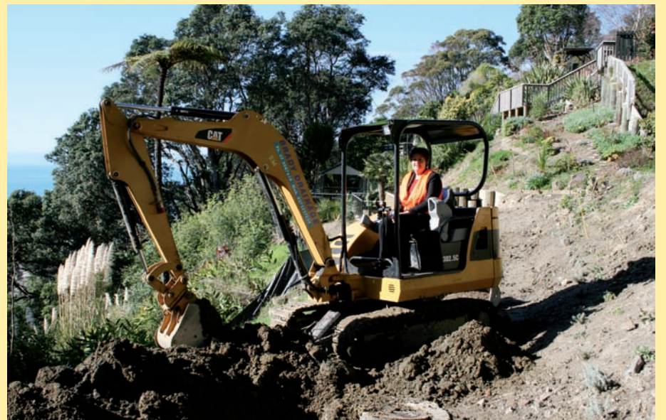
Done and Dusted! Whakatane District Council Chief Executive Diane Turner turns the last sod to mark the successful completion of the Otarawairere/West End reticulation project.
