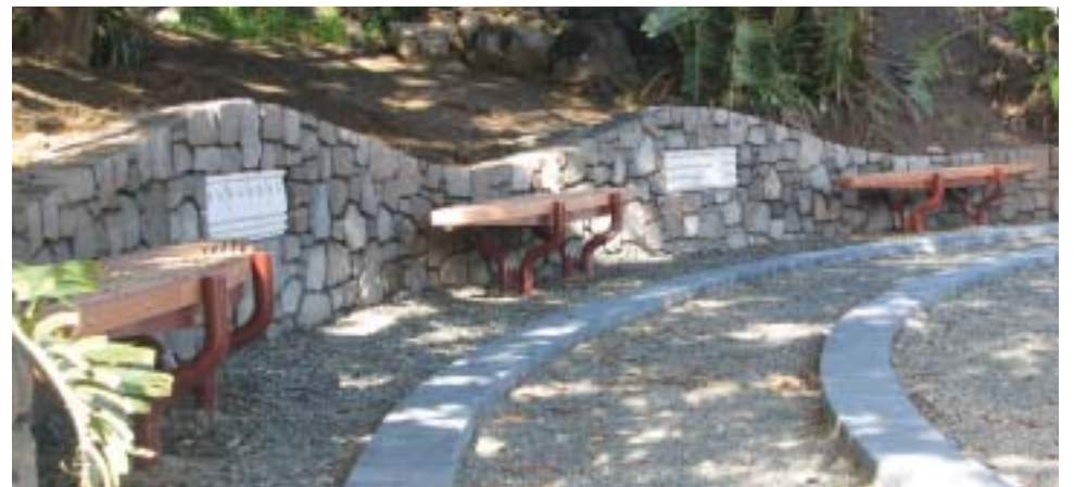
Work on the Commerce Street upgrade is on schedule. Installation of retaining wall and benches at Puketapu toe is now almost complete.
