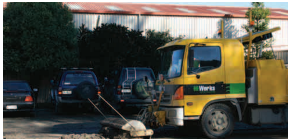
Road cleaning after the recent floods in Whakatane.
