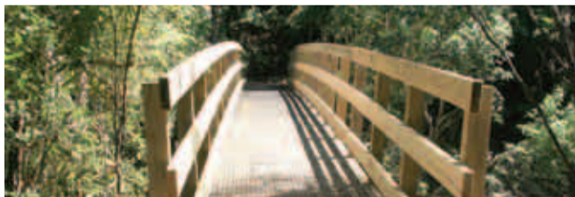
The new Bird Walk foot bridge was completed in time for Toi's Challenge early this month. It replaces the old bridge damaged in the June floods.
