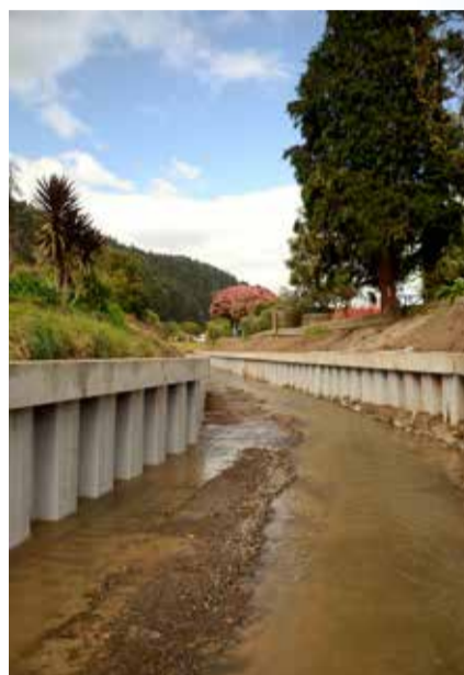
Sheet piling walls under construction on a 140m stretch of the Wainui Te Whara stream near Valley Road.
