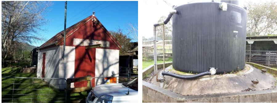
Figure 6: Rūātoki Treatment Plant housing UV Unit and Chlorine Cylinders (Left) and Holding Tank (Right)
