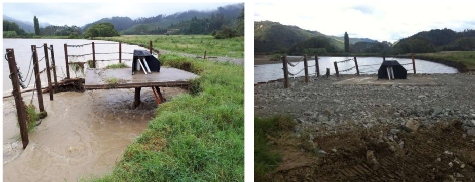
Figure 5: Bore Head at height of February 2018 floods (Left) and Emergency works underway (Right)
