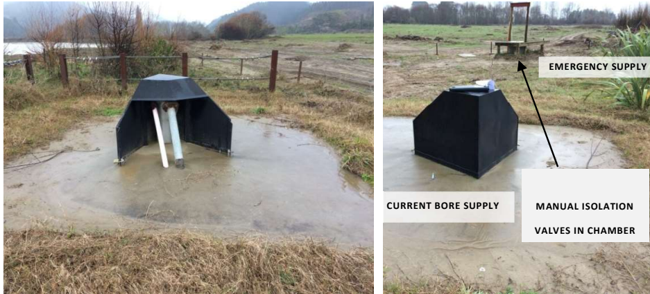
Figure 4: Bore Head with Steel Log Deflector (Left) and Emergency Supply and Isolating Valves (Right), prior to February 2018 River Intrusion
