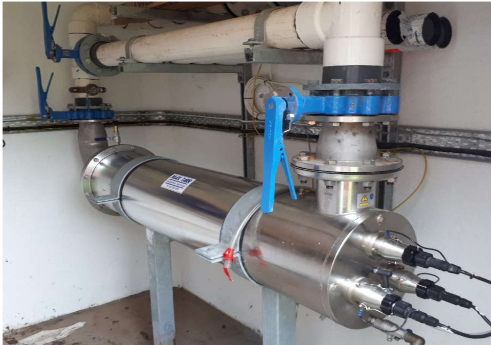
Figure 7: Ultra Violet Disinfection Treatment
