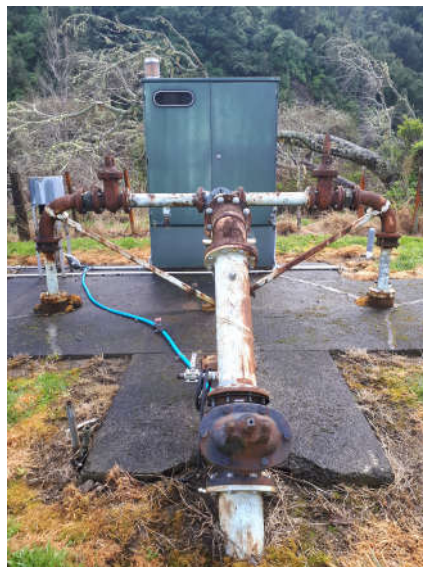
Figure 5: Bore Heads and Electrical Cabinet
