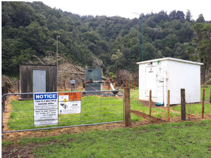
Figure 4: Bore Heads, Electrical Cabinet at Pump Station/Treatment Plant Site
