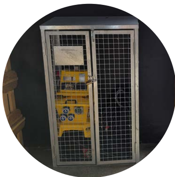
Locked cage containing external power equipment.
