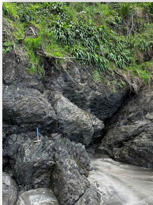
Photo 4: Strong bedrock at the base of the slip scarp.
