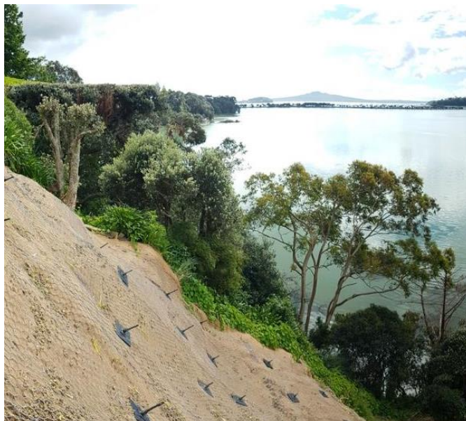
Figure 6: Rock anchor and mesh at top of slope to prevent future ground movement
