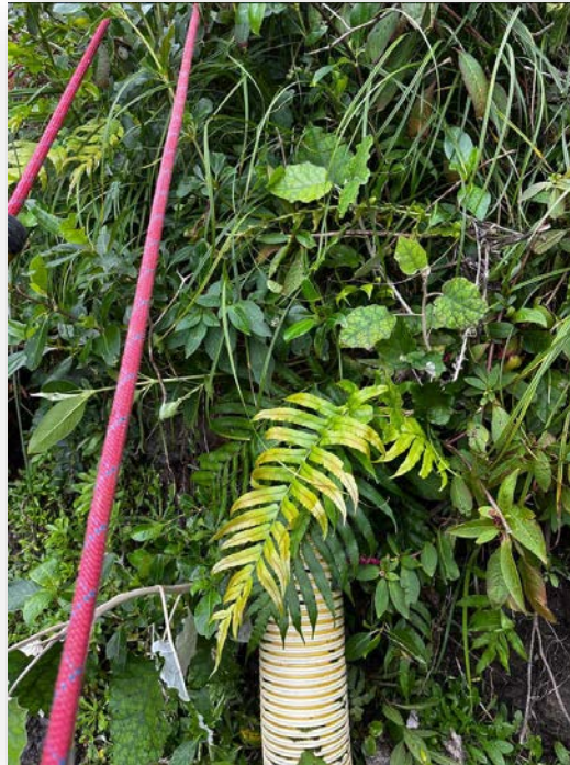
Photo 17: Old subsoil pipe above the original track alignment.
