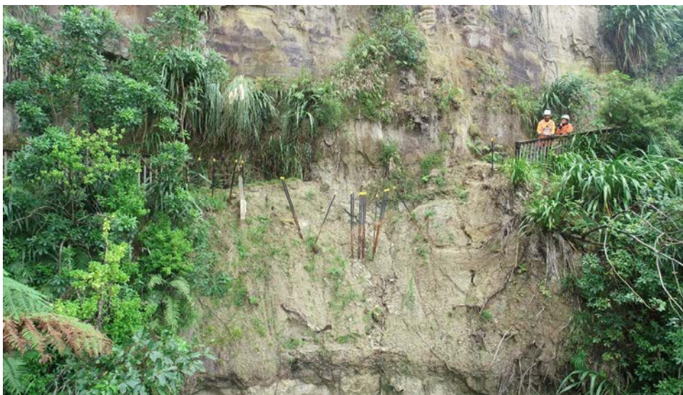
Underslip at Slip Area 2 – note most surface material has slid off exposing the sandstone underneath. Future failures are more likely to occur within the sandstone along the joints and other defects as part of more larger landslide event. Further failures are more likely to occur on either side of the existing failure due to similar shallow soils overlying the sandstone below.
