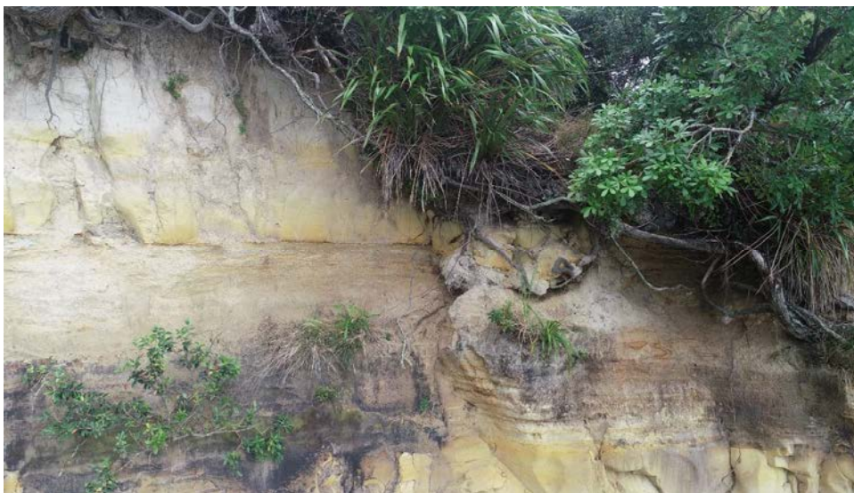
Right of face above Slip 2 track typical conditions – overhanging foliage, roots and sandstone blocks
