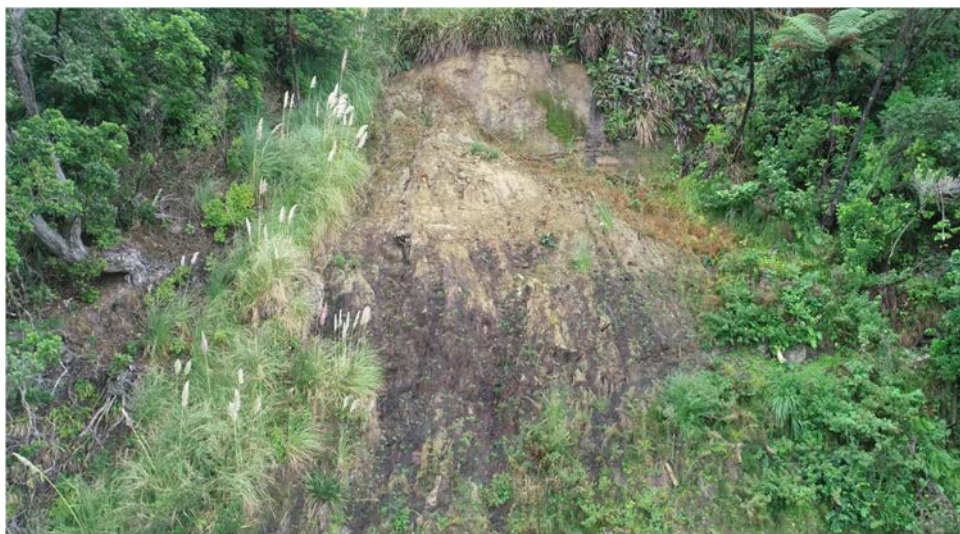
Overview of the upper section of slip 1 – The remaining track is visible by the yellow pipe on the right. The light coloured area at the top is the location of the recent slip with the older weathered face in grey below. Some residual soil and rock remain on the left where the Toitoi is growing, this is more likely remnant slip debris from an older event evident from the margins on the left and right of this slip.
