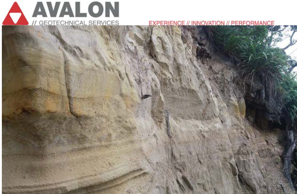
Right of the face above Slip Area 2 typical conditions – overhanging foliage, roots and sandstone blocks, note vertical joint exposed by the previous landslide.
