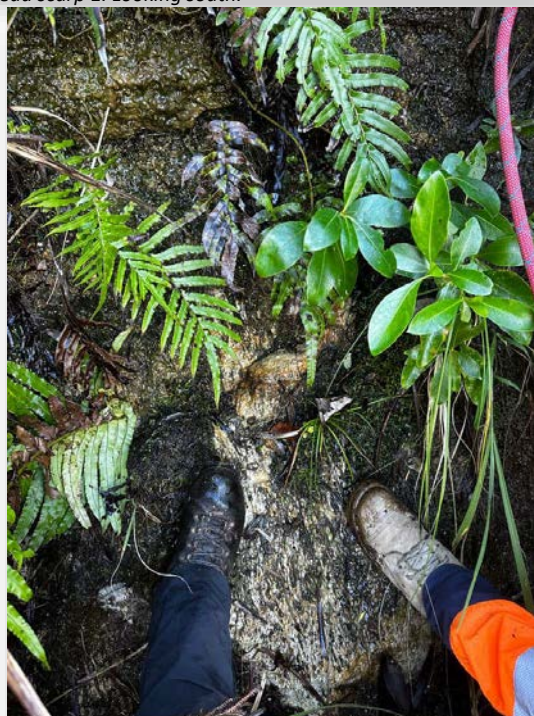
Photo 8: Between head scarp 1 and 2. Ground water seepage and algae.
