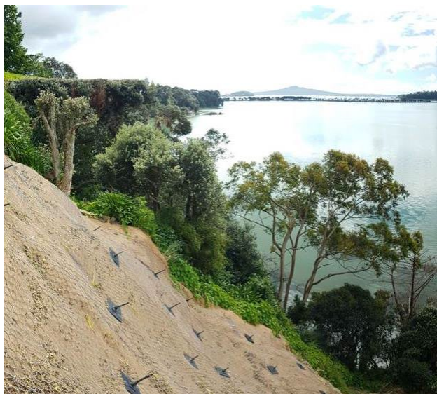
Figure 6: Example of rock anchors and rock mesh at the top of a slope to prevent future ground movement
