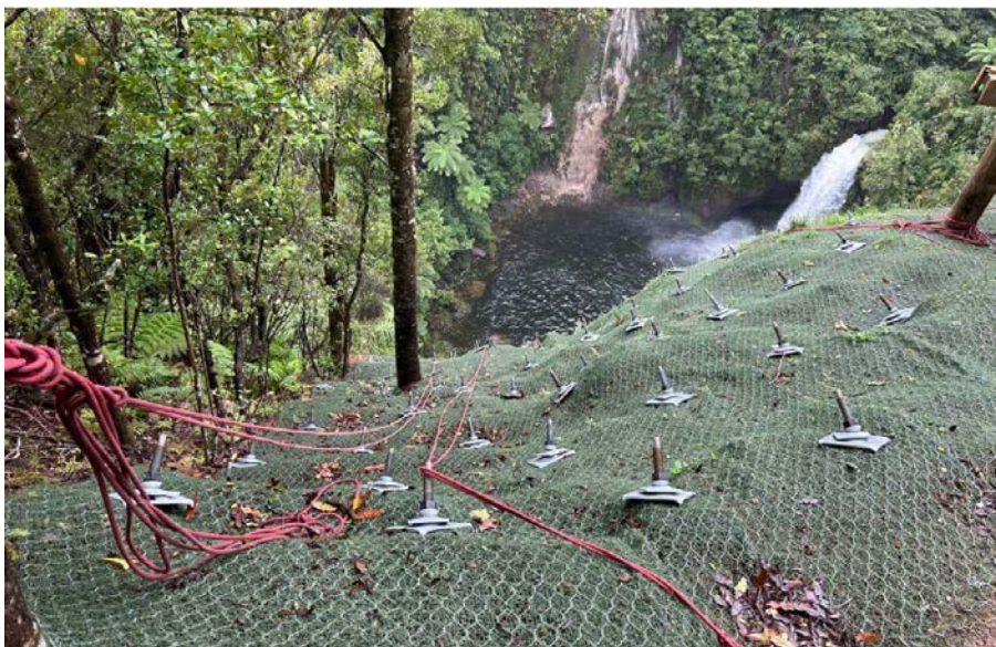
Figure 12.1: Photograph of anchorages and Mac-Mat-R mesh at Omanawa Falls during construction. (Source: T+T).
