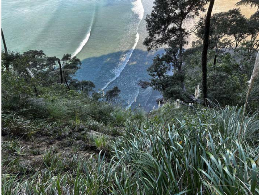
Photo 9: Looking down the landslide from slip scarp 3.
