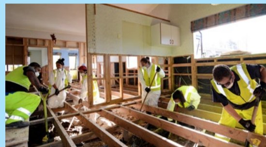
SHL contractors lifting up floorboards to clear the silt and mud build-up under homes affected by the Edgecumbe floods.
