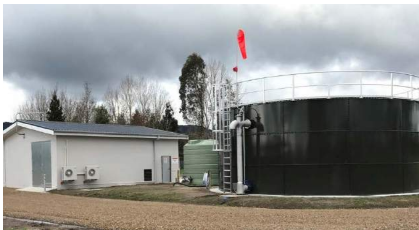
The Otumahi water supply scheme was commissioned in 2018 improving supply to Edgecumbe, Te Teko and parts of the Rangitāiki Plains.
