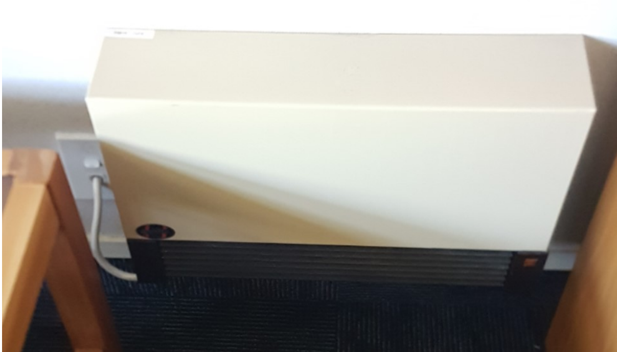
Figure 8-6 - Wall mounted 3kW electric heater at the Civic Centre
