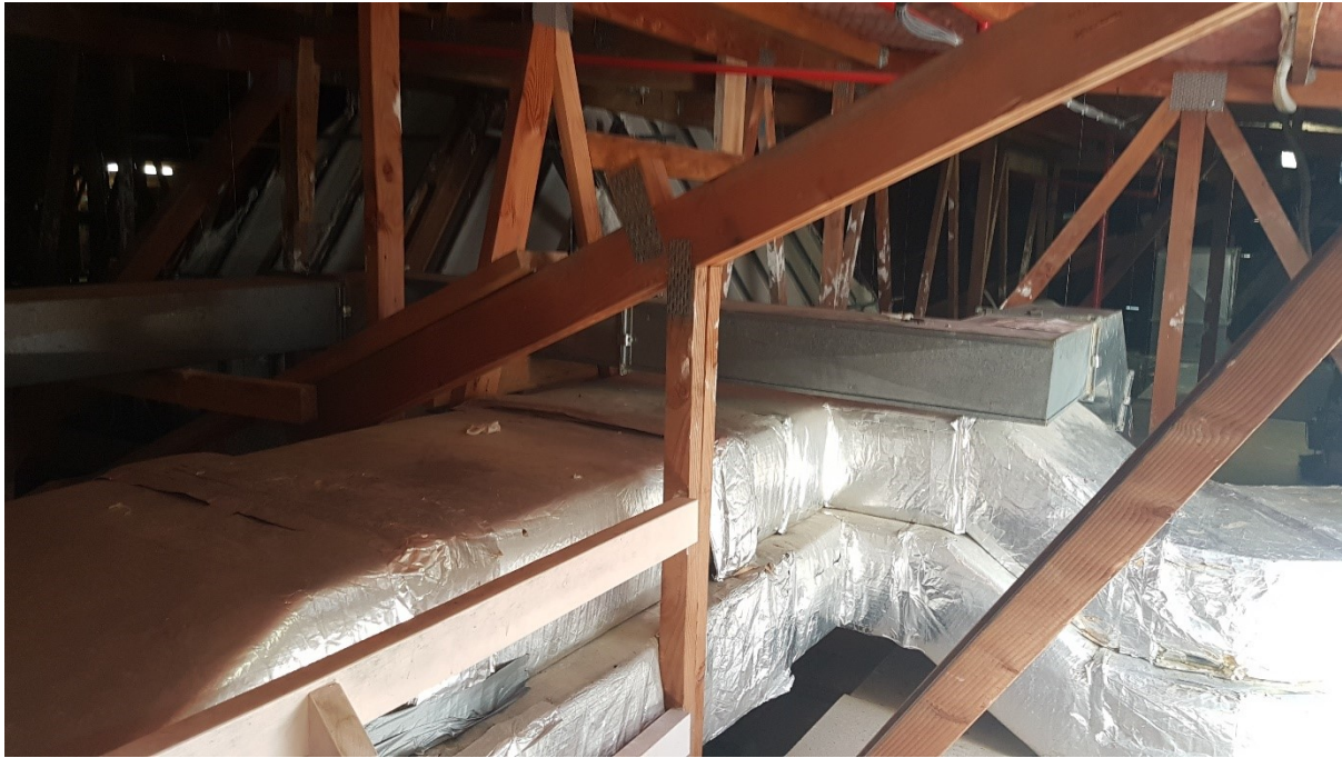
Figure 8-7 - Civic Centre roof-space showing there is no insulation on the second-floor ceiling, but there is on the underside of the roof.
